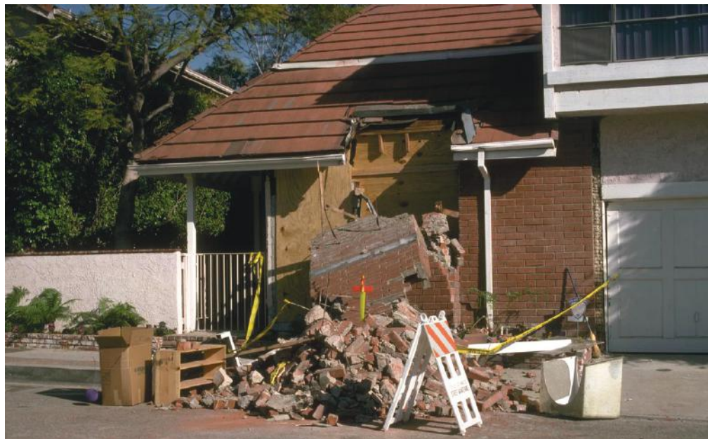
House devastation from the 1994 Northridge earthquake. Source: USGS
